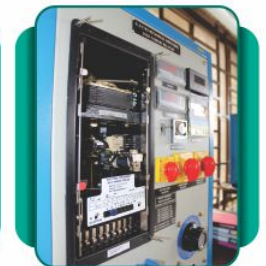
Switch Gear & Protection Lab
